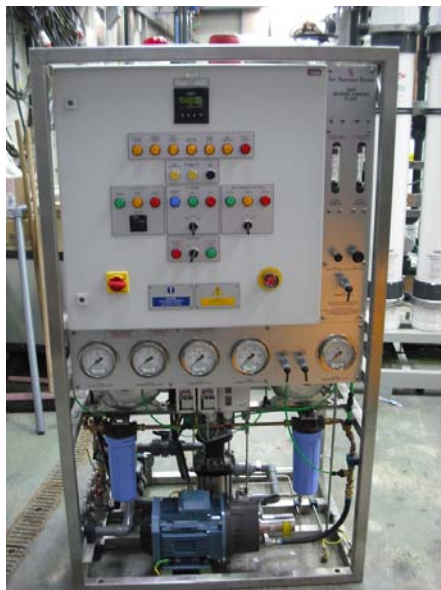
Technical Water RO Plant
