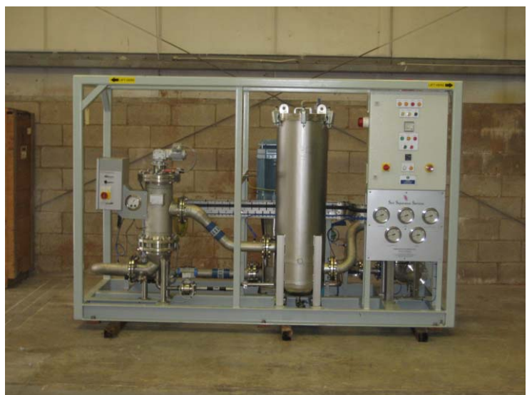
Fresh Water Embarkation Filter Unit
